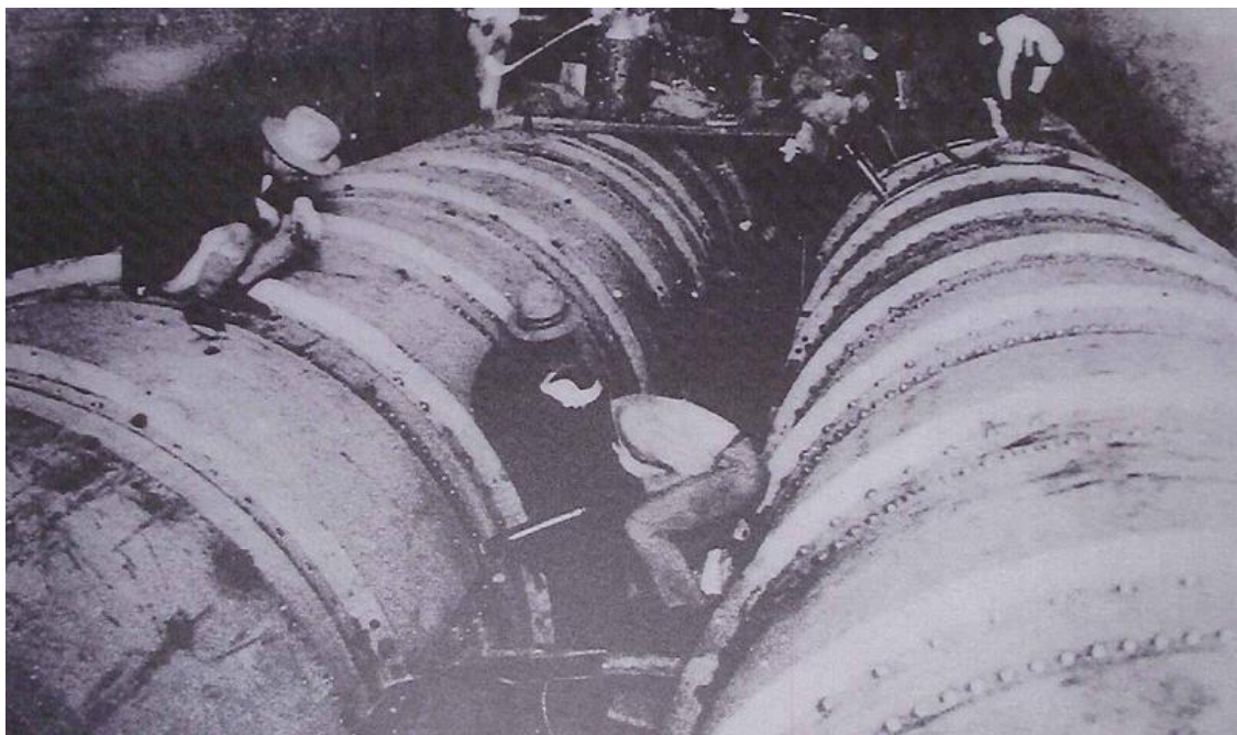
Figure 13: Riveting work for the iron pipes connecting the Sonnun-kei river with the Kandem-kei river to fill the water in the Uzanto-dam lake.
