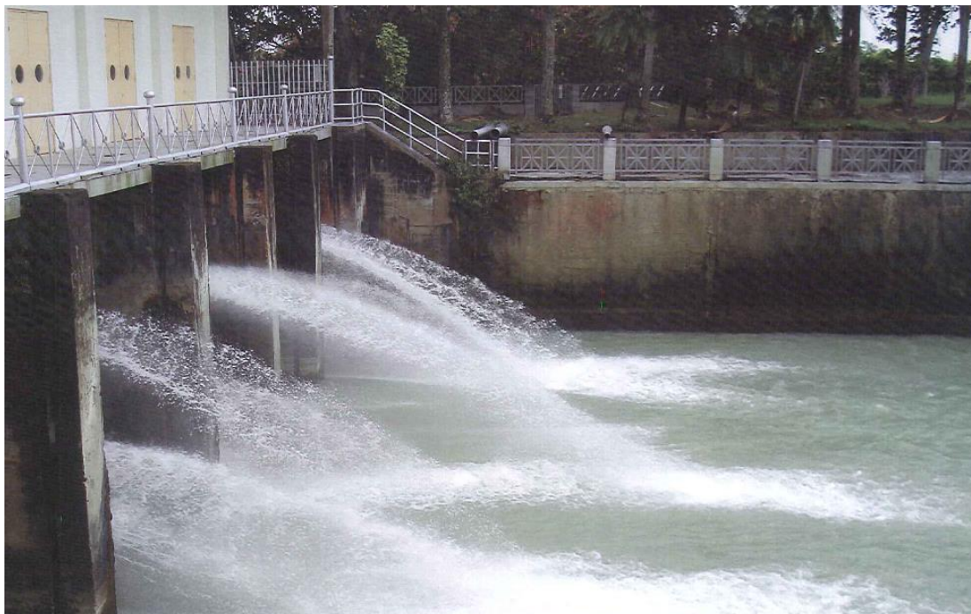
Figure 11: Discharge from the conduit exit through the Uzanto-dam bank.
